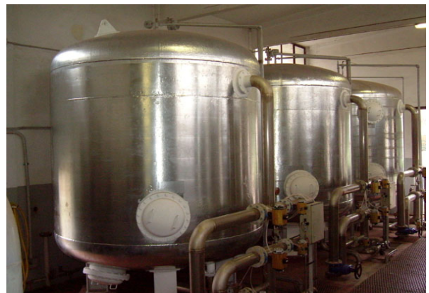
Condition of Tanks after ZincTape Application
