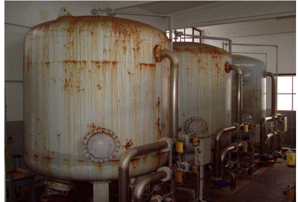
Condition of Tanks before ZincTape Application
